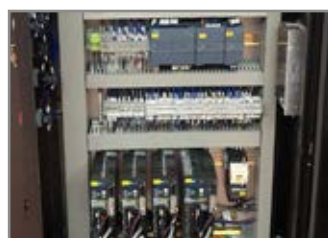
MACCHINA GESTITA DA PLC MACHINE CONTROLLED BY PLC
